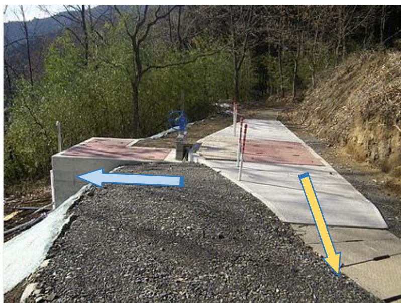
Figure 1: Irrigation channel/Intake/Forebay tank
