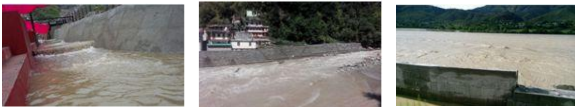
Performance of Defense Structures at Kedarnath, Kalimath and Srinagar, Uttarakhand
