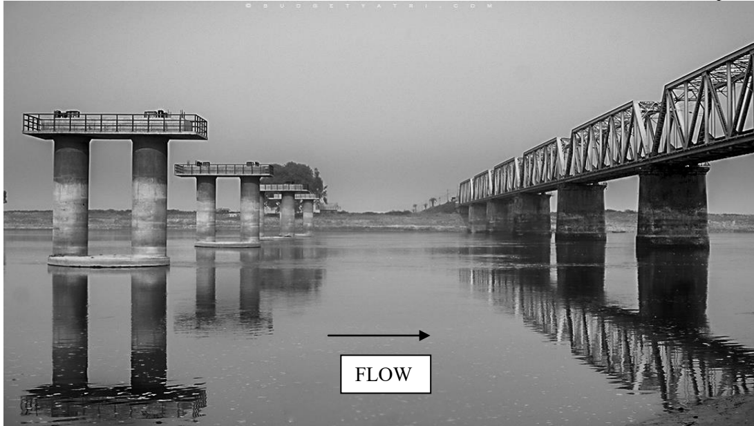
Figure 4 : Proposed bridge (under construction) on upstream side of existing bridge. (View from Katareah end)
