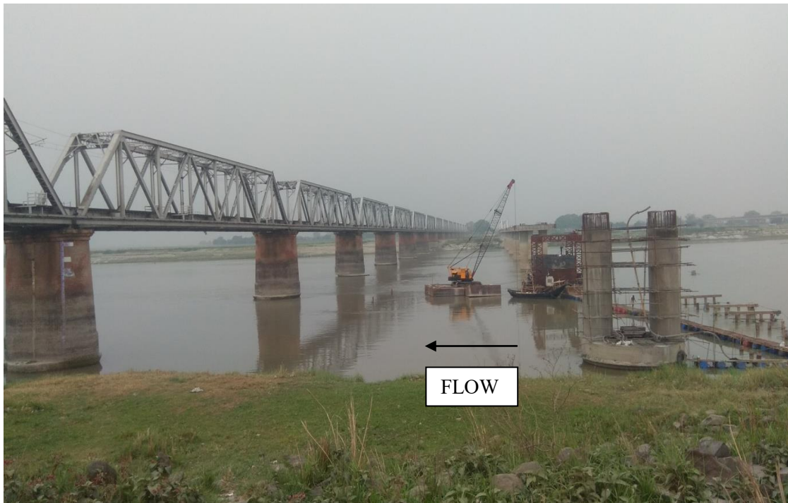
Figure 5: Proposed bridge (under construction) on upstream side of existing bridge. (View from Kursela end)
