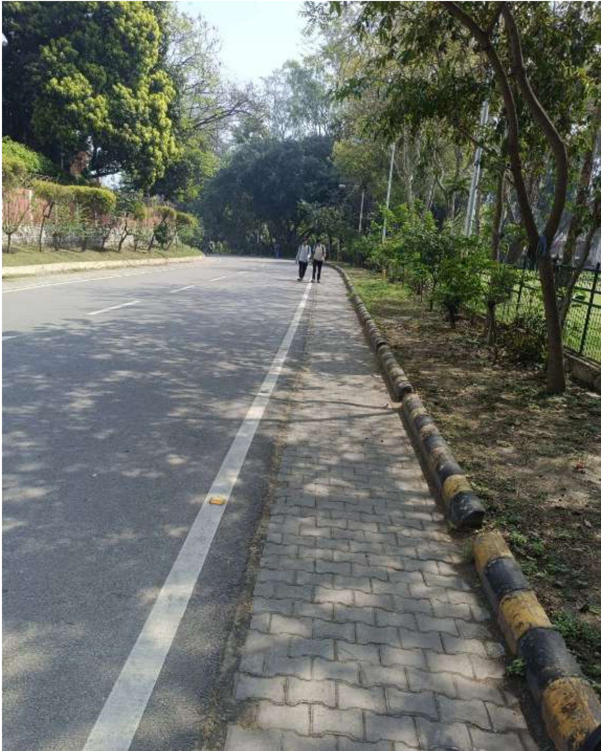
Figure 7 Surface restoration (removal of paving) along the road along WRDM and NC Nigam
